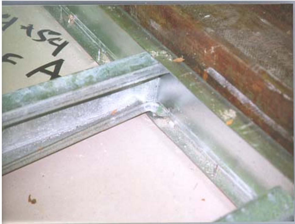
FIGURE 7 Failure of a 2x4x54 mil wall stud by crippling at the end of the stud with 0 psf lateral load (sheathing has been removed).
