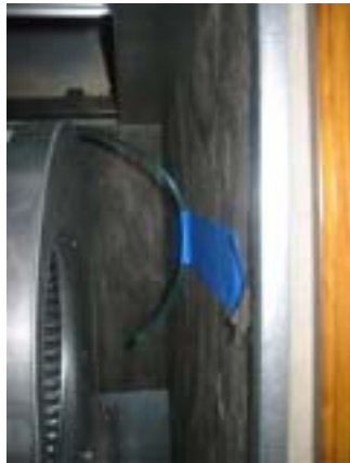
Figure 2-5 Pressure probe at air handler fan
