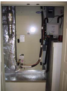
ZEH-HVAC Air Handler
