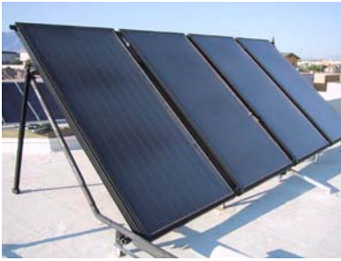
ZEH-Solar Thermal Collectors
