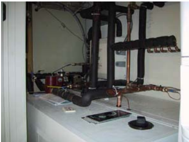
ZEH-Hot Water Storage
