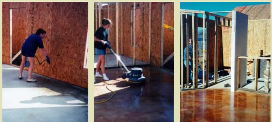
From left to right: First stain coat applied, sealant is applied and buffed over stain coats, finished floor, Carl Franklin Homes Field Evaluation
