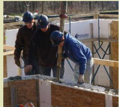
Three students help fill ICF forms with concrete; LCCTC Lancaster PA Field Evaluation
