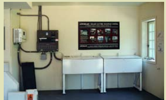
PV Power storage batteries
