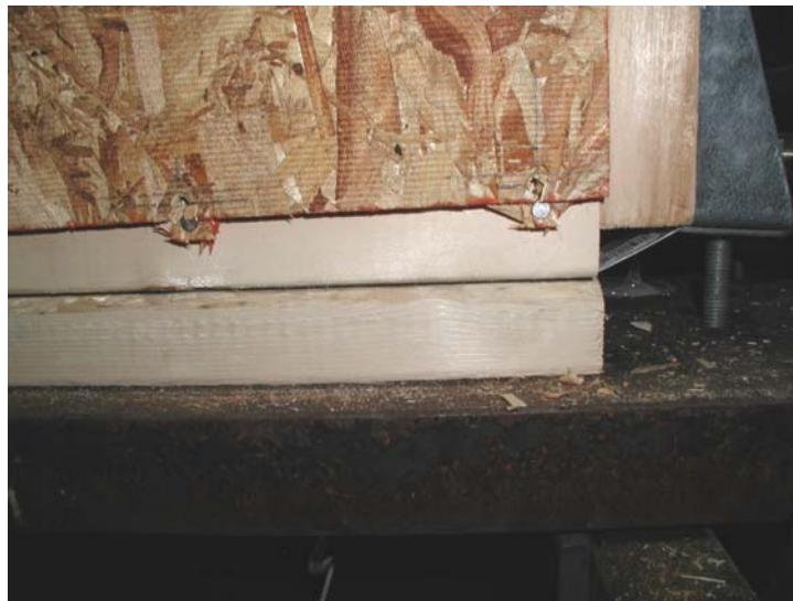
Figure 3.6 – Fastener tear-through failure at region D
