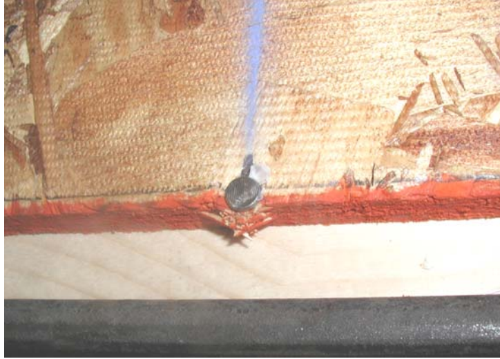
Figure 4.1 – Ineffective nailing for “Edge Distance #3”
