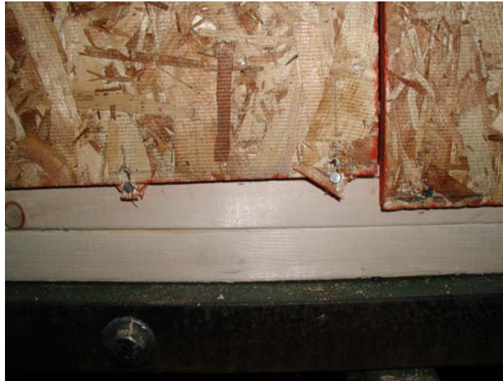
Figure 3.8 – Fastener tear-through failure at region F
