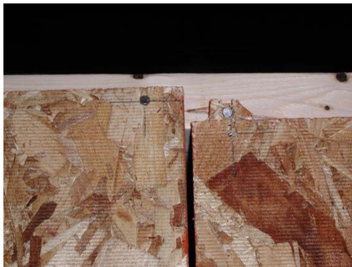
Figure 3.9 – Fastener tear-through failure at region G
