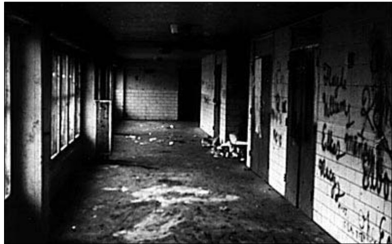
Figure I-3: The 3d floor communal corridor as it actually turned out, showing the vandalism that ensued.
