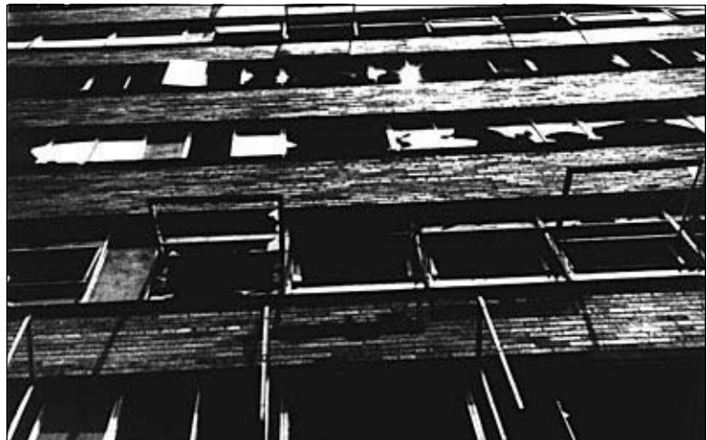
Figure I-4: Vandalism to the large number of vacant apartments in Pruitt-Igoe as seen from the outside.
