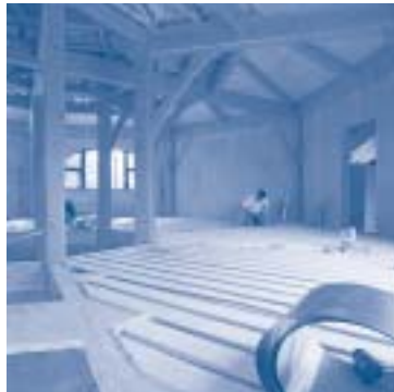
Contractors install PEX tubing for a radiant flooring system prior to installing the finished floor
