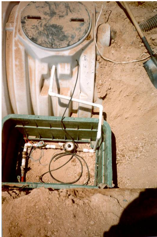
Figure A6 Tap water supply to the rainwater storage tank showing the research center water meter, solenoid valve, and manual shut off valve.
