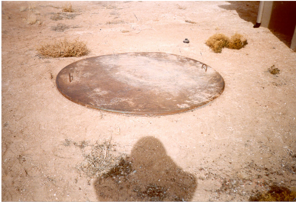
Figure A1 Steel cover for gray water system underground pit.
