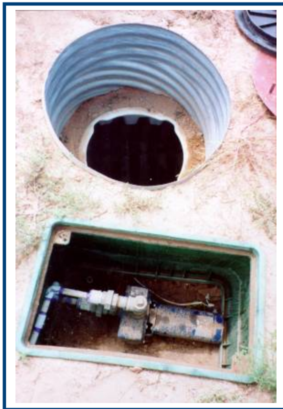
Figure 11 The rainwater collection tank has a ground level access hatch adjacent to the pump
