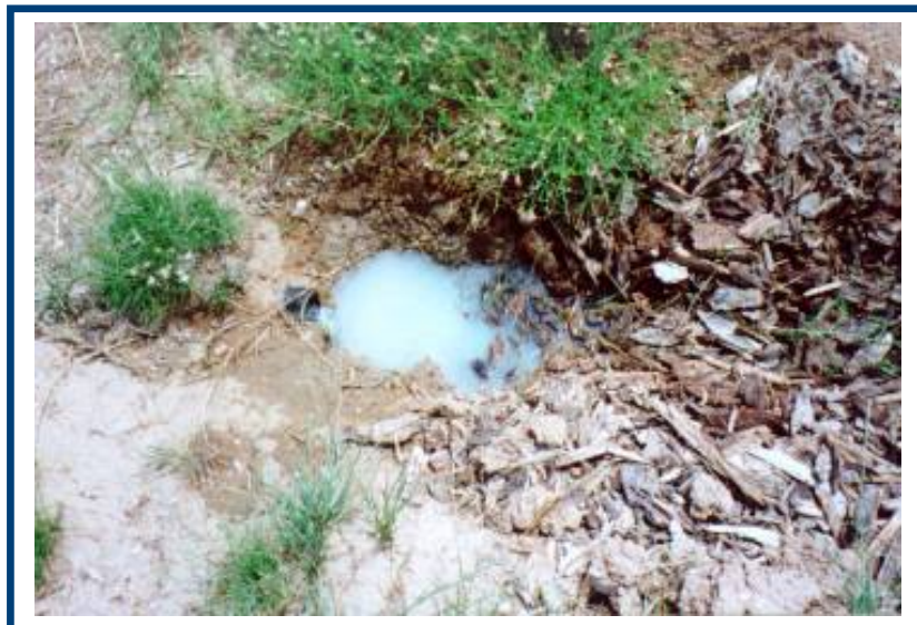
Figure 7 Gray water outlet located in a mulched area. (Uncovered for photo)
