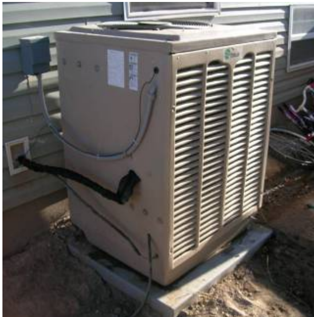
Figure 2. Freus Evaporative Condenser (Unit A)
