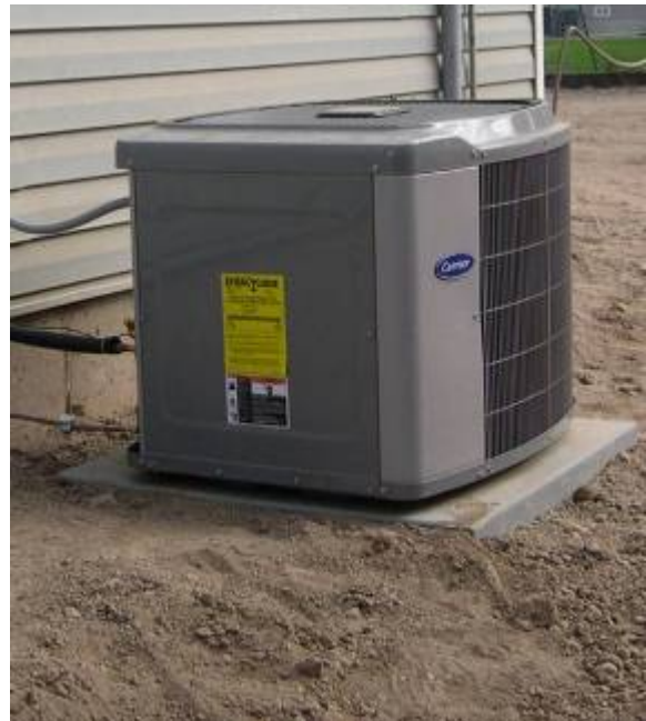
Figure 3. Air Cooled Condenser (Unit B)
