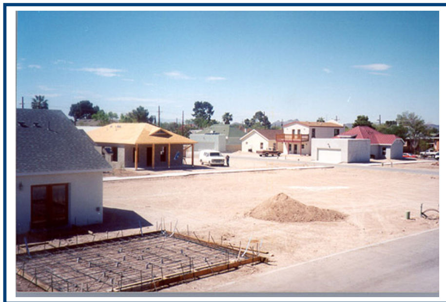
Figure 4: Homes under construction at Armory Park del Sol (model homes in background)
