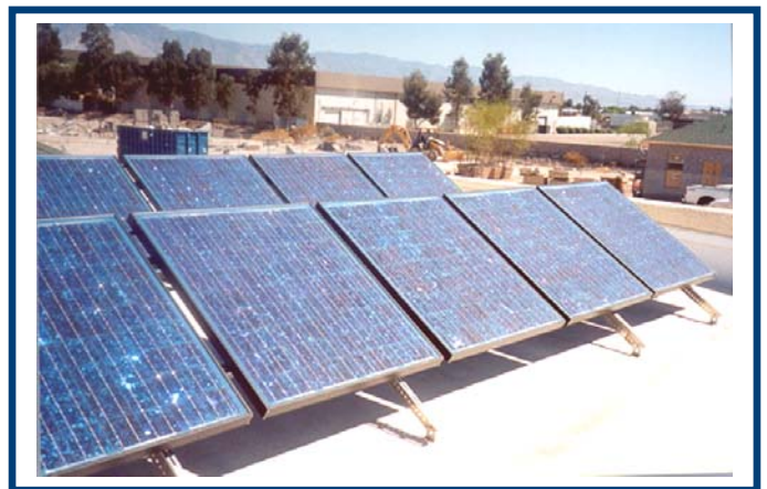
Figure 15: PV Array at House A
