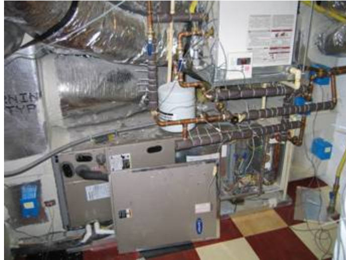
Figure 4. Short Term Monitoring Sensors
