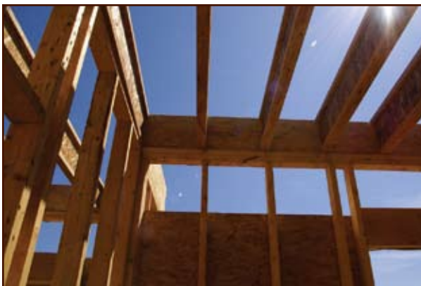
Stacked, or in-line, framing allows loads to be transferred directly downward and can eliminate the need for double top plates.
