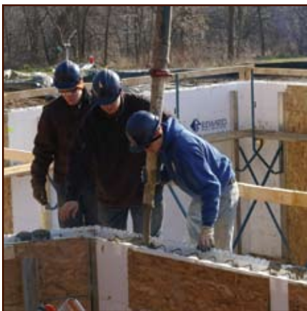
An insulating concrete form basement is an integral part of the energy-efficient building shell.
