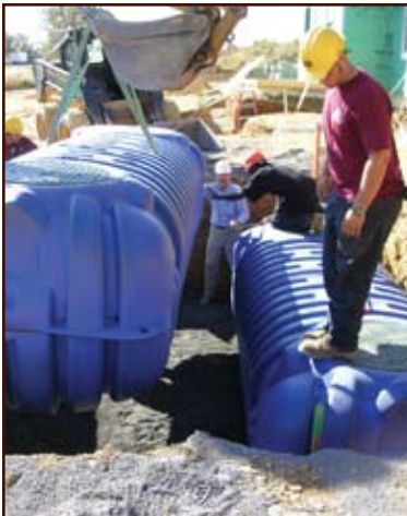
The rainwater harvesting tanks are placed on a gravel pad to be buried under ground.
